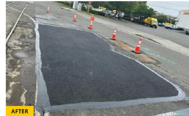
Sinkhole repair at Diagonal Ave S / Colorado Ave S / S Oregon St
