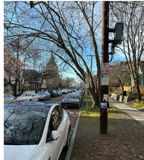
Existing curbside electric vehicle chargers.
